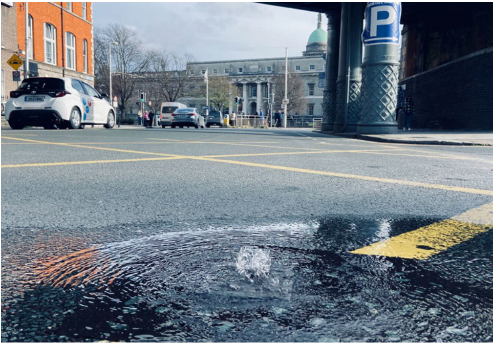
Water bubbling up on Lower Gardiner Street. Credit: Richard Carson
